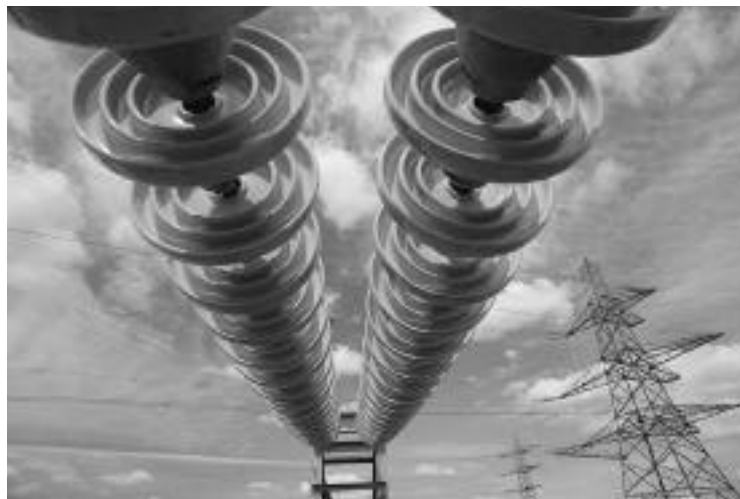
Communication between system control centers and monitors and sensors throughout the grid ensure a comprehensive understanding of power system conditions.
